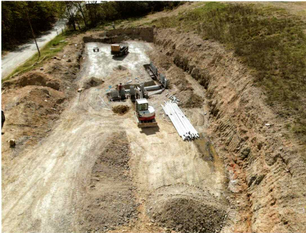
2500KW Generator Site - Davidson WWTP
